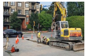
Continuing to set aside funds to replace civic buildings, utilities and other infrastructure
